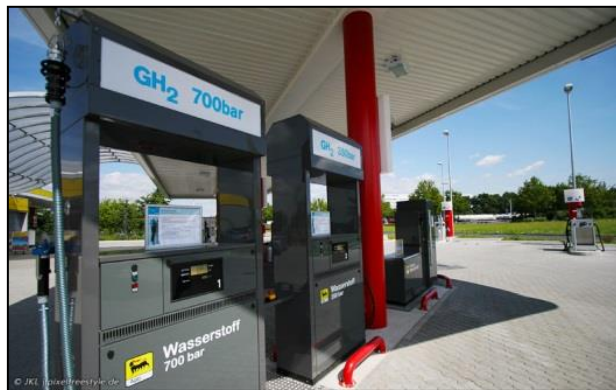
Photo 7: Hydrogen station in Höchst, district of Frankfurt am Main, Germany.
