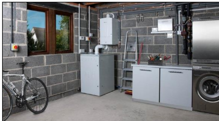
Photo2: BlueGen fuel cell installed in a home in Sheffield (Source: CFCL)
